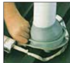
Step Four Form Press, bending flashing to fit irregularities. Use large slot screwdriver to press into tight angles.
